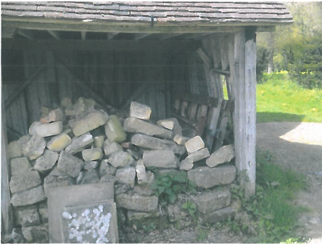
Damage to (right hand) flank / front corner
