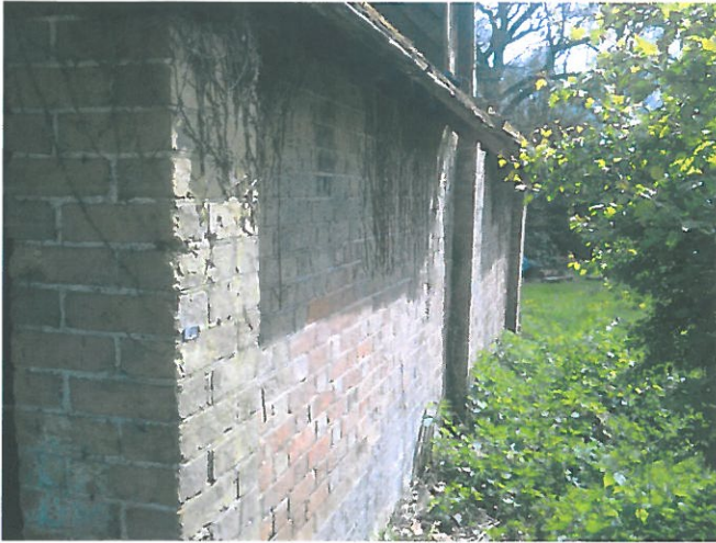
Overgrown vegetation side (South) section
